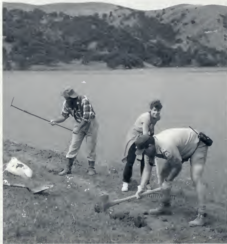
Each year, volunteers join park staff in trail construction and rehabilitation at various regional parklands. These workers are putting in a new trail at Del Valle Regional Park during the annual statewide Trail Days. Photo by Steve Fiala.
